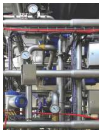
Example of ash slurry pumping systems
