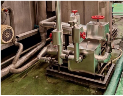
Steam-operated pump trap (SOPT) installed at Bottle Washer Line 4.
