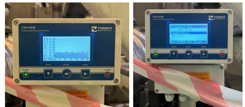
Steam-operated pump trap (SOPT) and a steam-operated pressure powered condensate recovery pump (PPPU) installed at Bottle Washer Line 5. The condensate recovery meter (CRM) shows totalised flow rate and temperature
