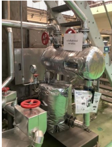
Steam-operated pump trap (SOPT) and a steam-operated pressure powered condensate recovery pump (PPPU) installed at Bottle Washer Line 7. The condensate recovery meter (CRM) shows totalised flow rate and temperature
