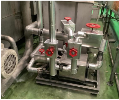
Steam-operated pump trap (SOPT) installed at Bottle Washer Line 6.
