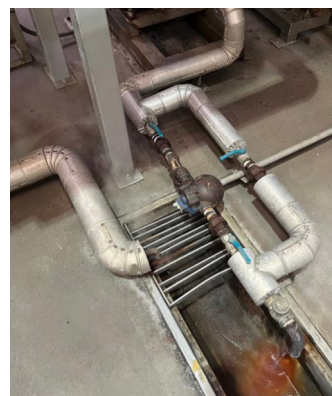
Stalling condition of the float trap at the PHE resulting in condensate being drained locally
