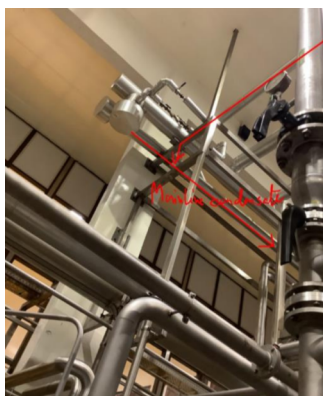
Condensate line lifted to a 5 meter height, causing backpressure on the float traps
